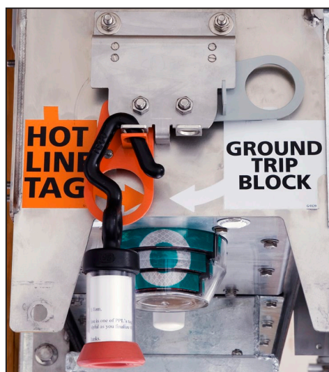
Figure 8. The Hot Line Tag mode manually applied and “tagged.”
