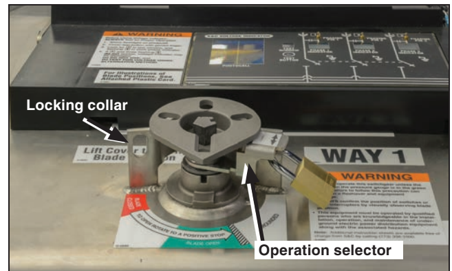
Figure 26. Locked out of the Grounded position.
