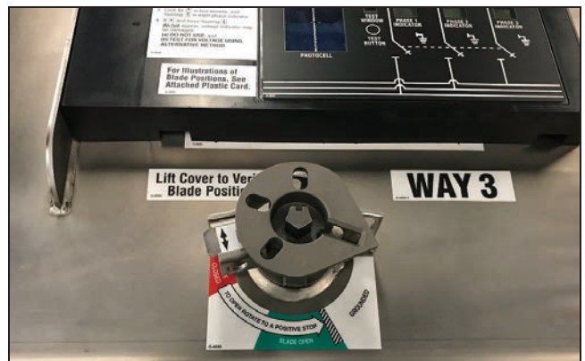
Figure 18. The load-interrupter switch or fault interrupter in the Grounded position.
