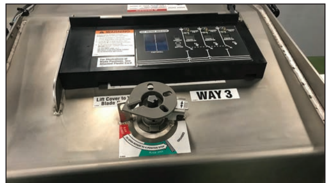
Figure 22. Load-interrupter switch or fault interrupter in the Closed position.
