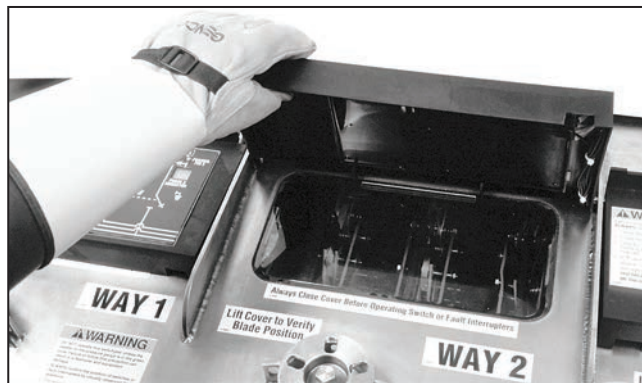
Figure 9. Window cover lifts for viewing of switch or fault-interrupter blade positions.
