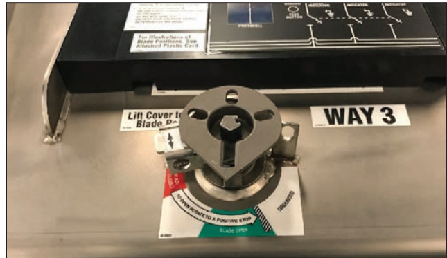
Figure 20. The load-interrupter switch or fault interrupter in the Open position.
