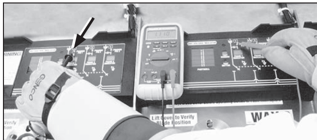
Figure 41. Measuring phase-to-phase voltage—Phase 1 to Phase 1.
