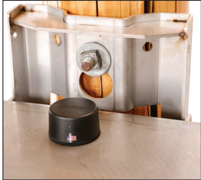
Figure 16. GPS antenna installed on the top of the IntelliRupter fault interrupter base.
