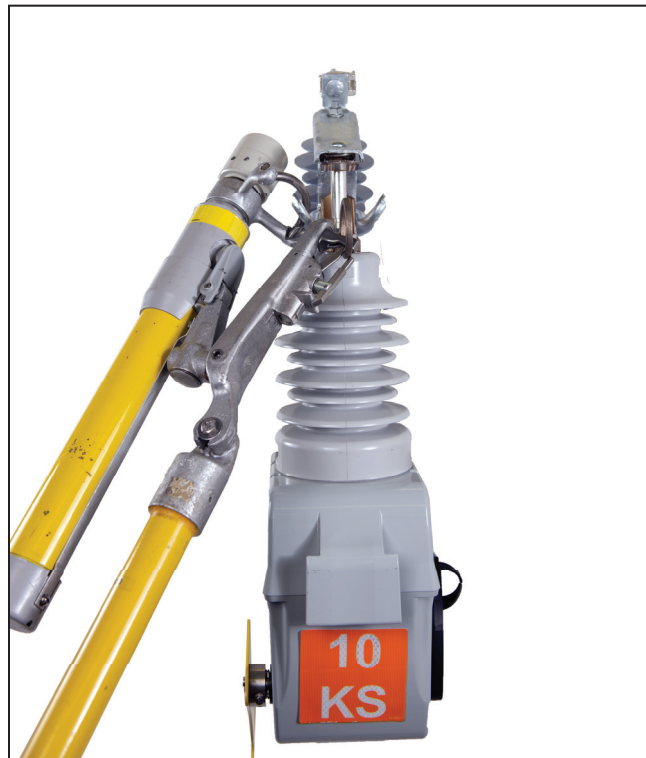
Figure 26. An incorrect fastening approach.
