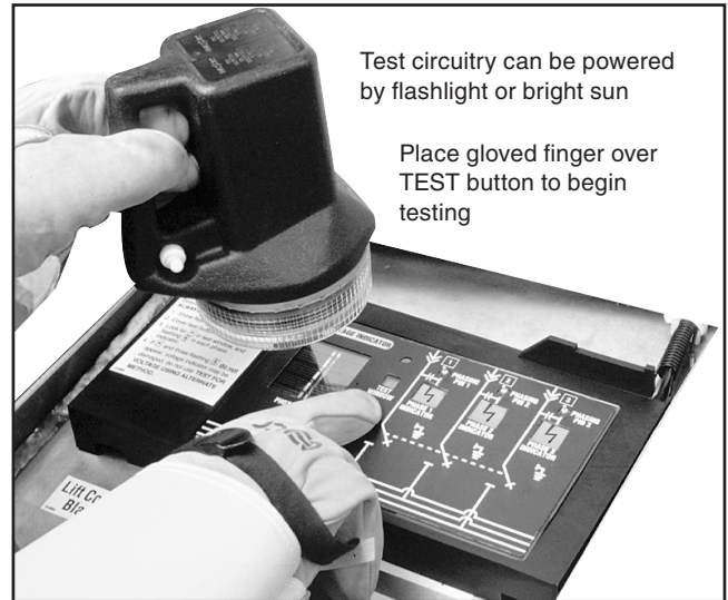
Figure 24. Testing the Voltage indicator.
