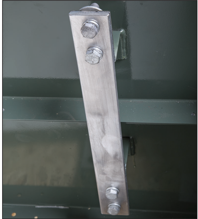
Figure 21. The enclosure ground pad.
