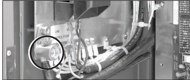
Figure 92. Copper lug and fuse block.
