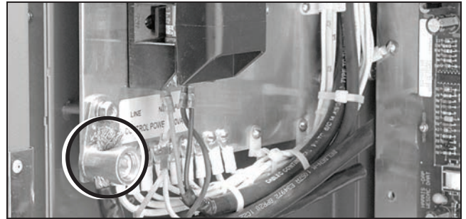
Figure 62. Copper lug and fuse block.
