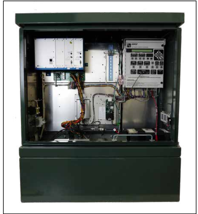
Figure 76. A vault-style low-voltage enclosure shown with a 6802 Automatic Switch Control and provision for communications.
