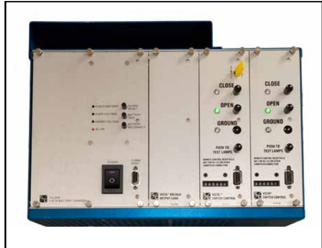
Figure 73. The Open indication on the motor control board matches the motor operator position.
