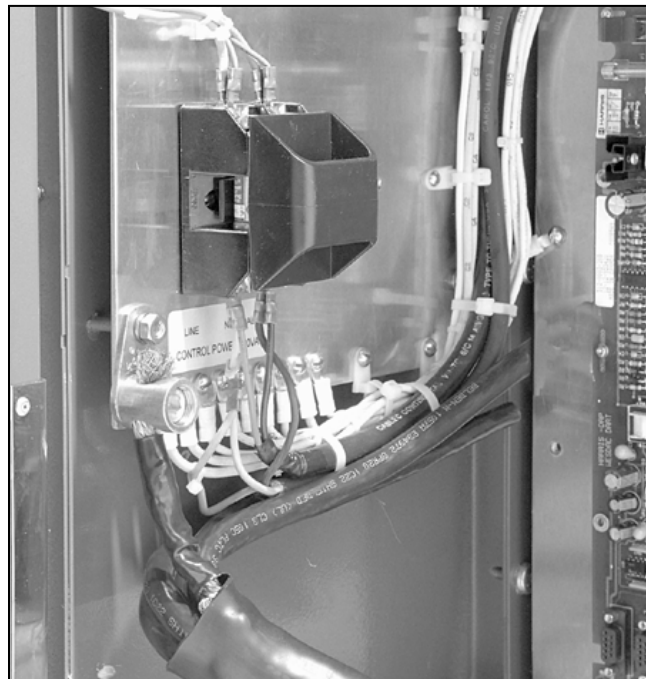
Figure 35. The fuse block.
