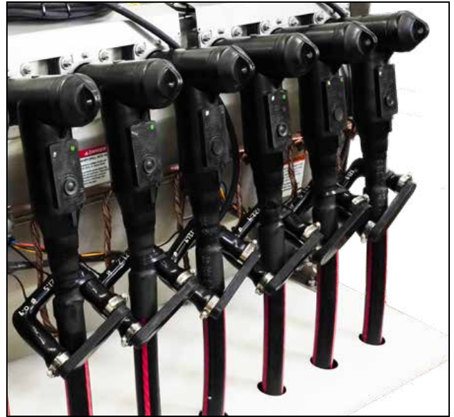
Figure 111. Wiring is already attached to the current sensors.
