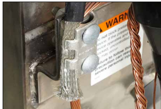
Figure 110. The shielded cable connected to the tank ground.
