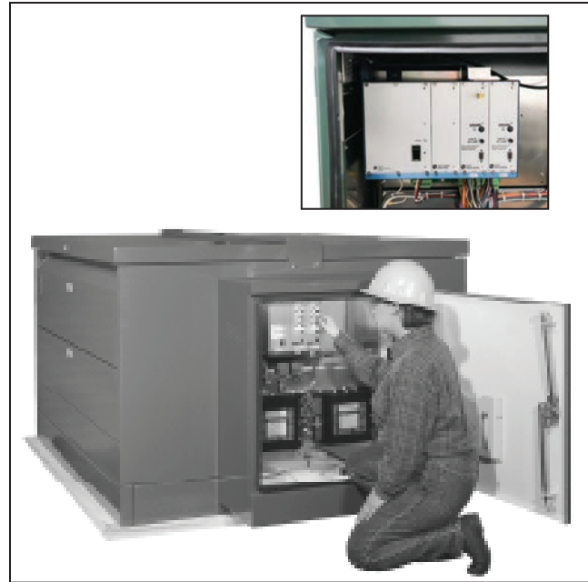
Figure 39. The location of the motor operator controls.
