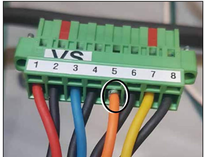
Figure 32. An example of an improper connection that is backed out.
