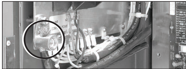
Figure 122. The copper lug and fuse block.
