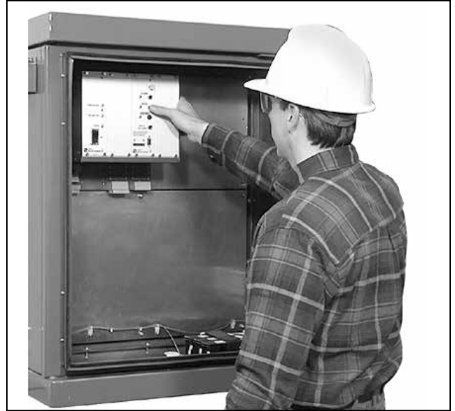
Figure 104. A vault-style low-voltage enclosure shown with provisions for a remote terminal unit and communications.
