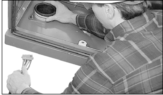
Figure 118. Inserting the cables into the low-voltage enclosure via the tubing and conduit.
