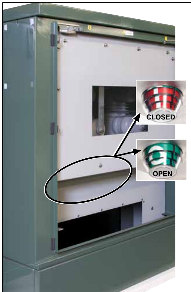
Figure 11. The Interrupter fault interrupter OPEN/CLOSED indicator, one at each pole. A red target with an “I” shows the interrupter is closed; a green target with an “O” shows the interrupter open.
