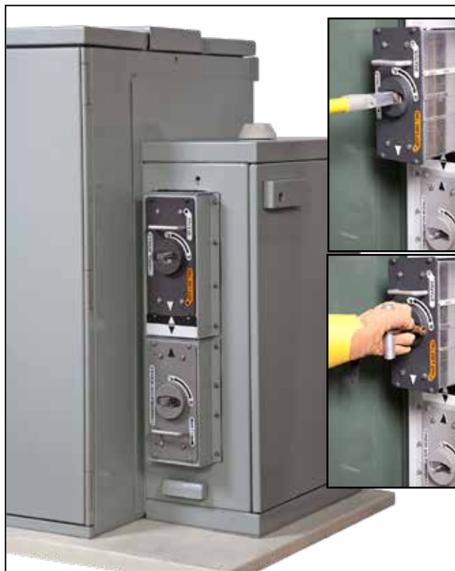
Figure 9. The protection and control module (top) and communication module (bottom) installed in the low-voltage compartment.
