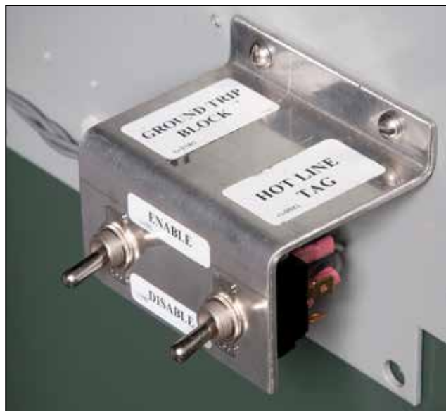
Figure 15. The HOT-LINE TAG and GROUND TRIP BLOCK toggle switches. The features are enabled when the switches are in the Up position.
