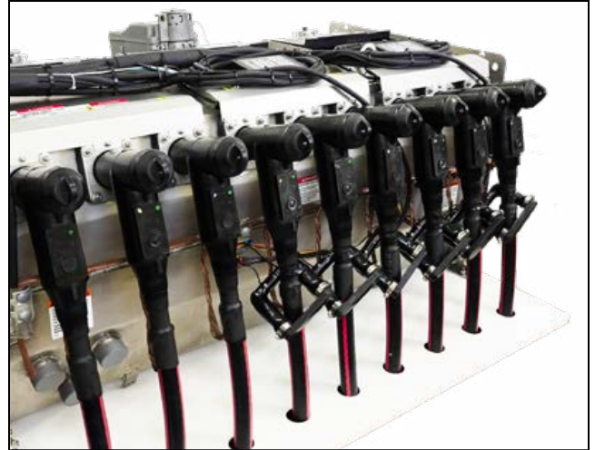
Figure 113. The wiring is already attached to the current sensors.
