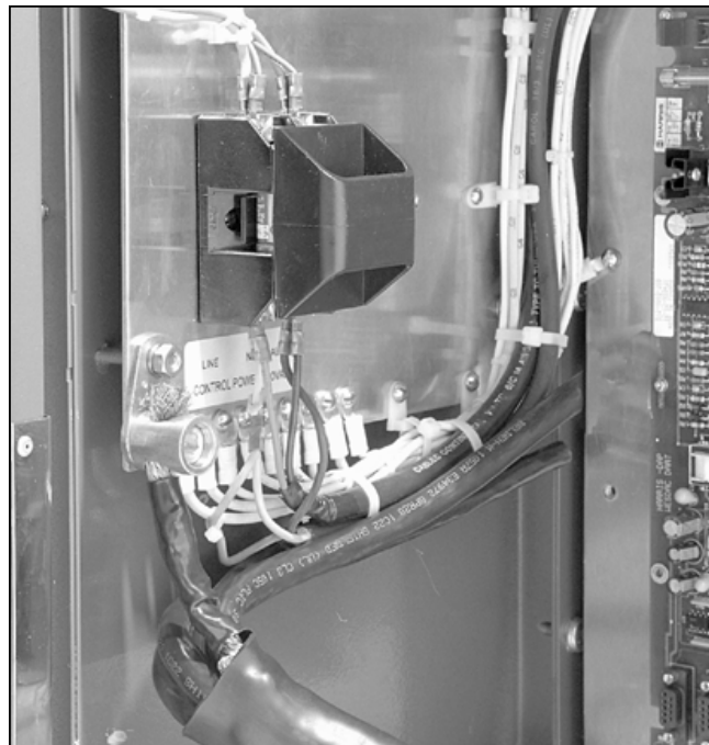
Figure 35. The fuse block.
