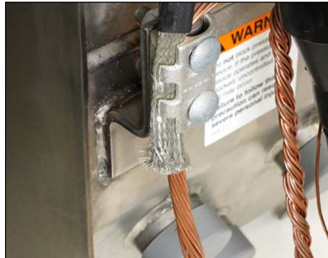
Figure 112. The shielded cable connected to the tank ground.
