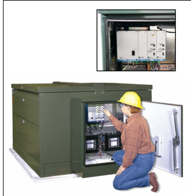
Figure 46. The location of the motor operator controls.
