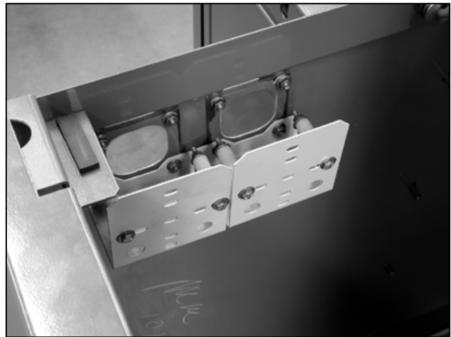
Figure 24. The mounting brackets for user-furnished fault indicators.
