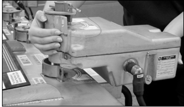
Figure 126. The motor operator placed over the operating shaft on the gear.
