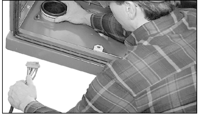
Figure 90. Inserting the cables into the low-voltage enclosure via the tubing and conduit.
