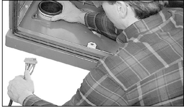
Figure 120. Inserting the cables into the low-voltage enclosure via the tubing and conduit.
