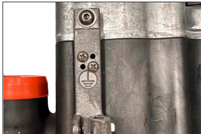
Figure 44. The bushing well interrupter grounding point marked with the "earth ground" symbol.
