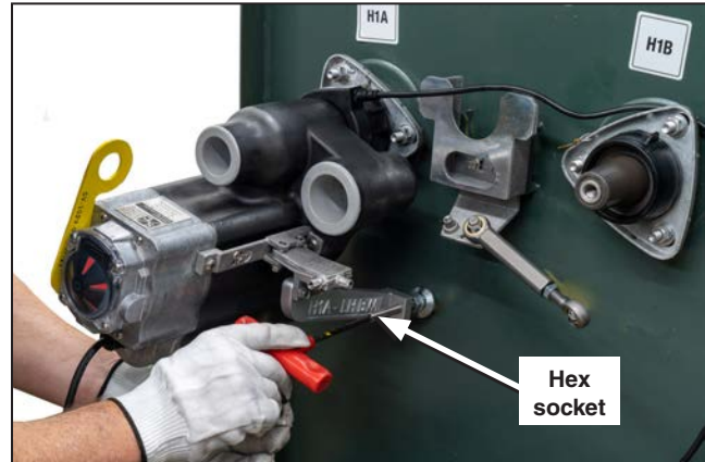
Figure 21. The hex socket at the top of the H1A bushing well interrupter swivel foot.
