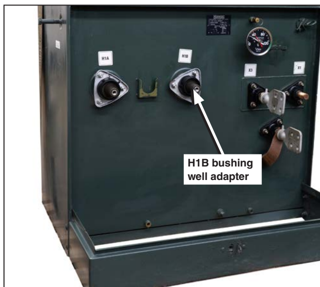
Figure 7. Installed bushing well adapters.
