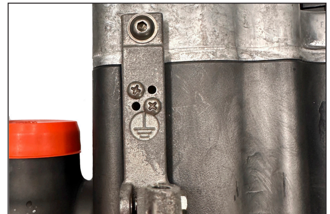
Figure 34. The bushing well interrupter grounding point marked with the "earth ground" symbol.
