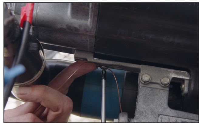
Figure 33. The bushing well interrupter grounding point.
