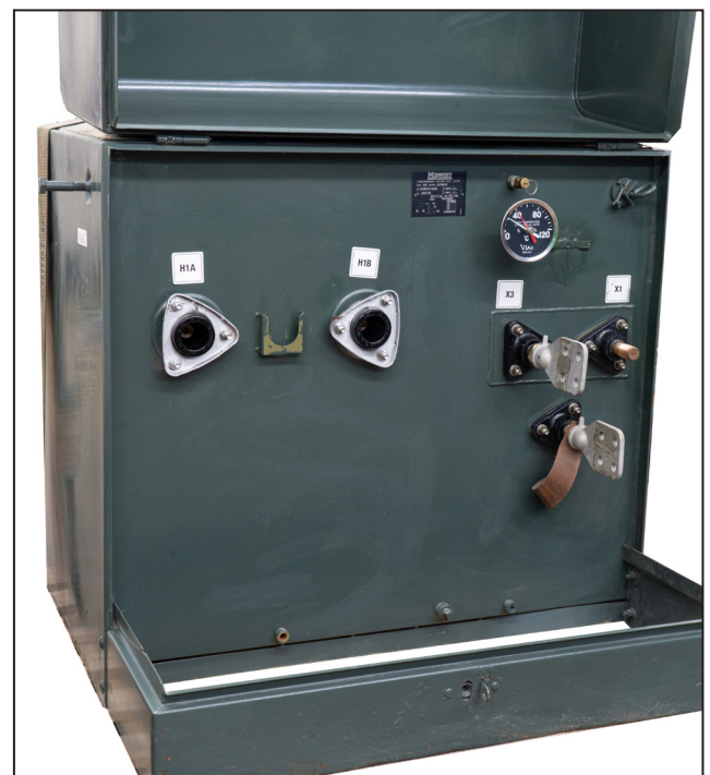
Figure 5. Bushing wells with loadbreak inserts removed.
