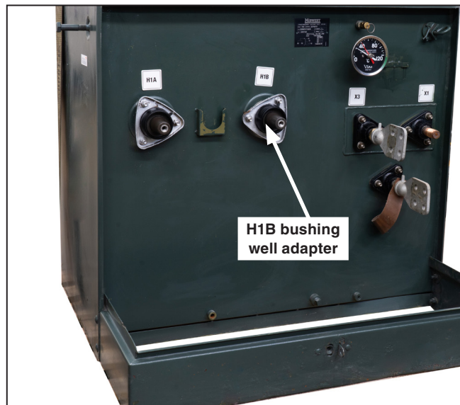
Figure 7. Installed bushing well adapters.
