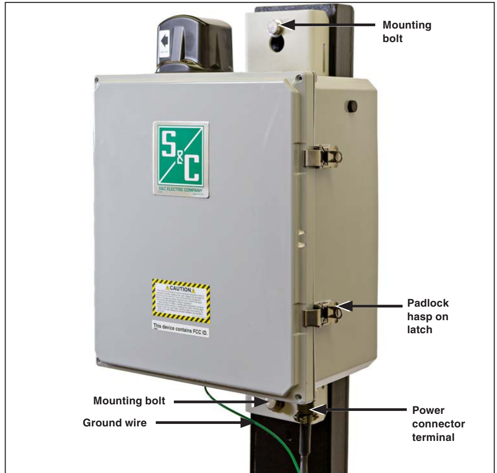
Figure 2. Mounting the communications gateway to the utility pole
