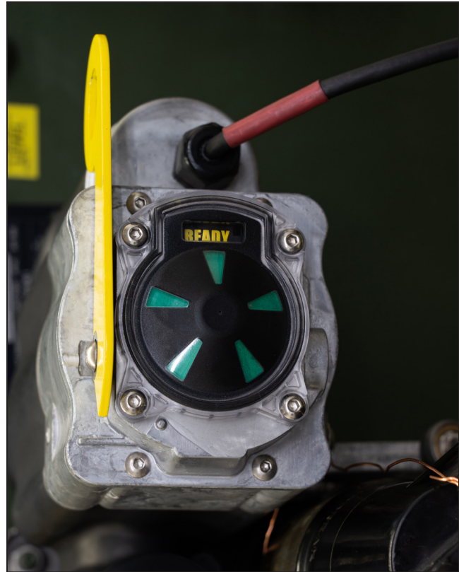
Figure 20. A bushing well interrupter in the Open and Ready position. In this position, automatic operation is enabled.
