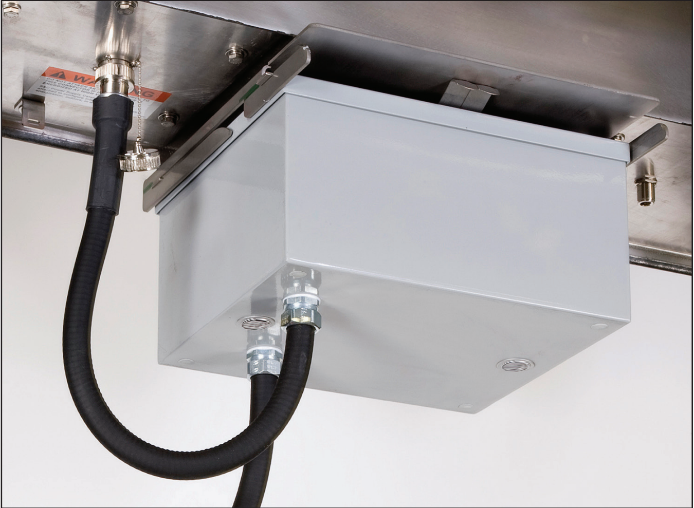
Figure 5. An external power supply connected to the IntelliRupter fault interrupter.
