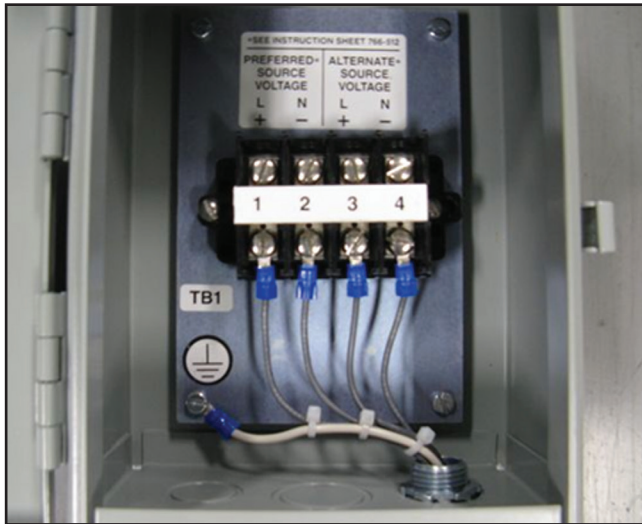
Figure 8. Junction box power input terminals.
