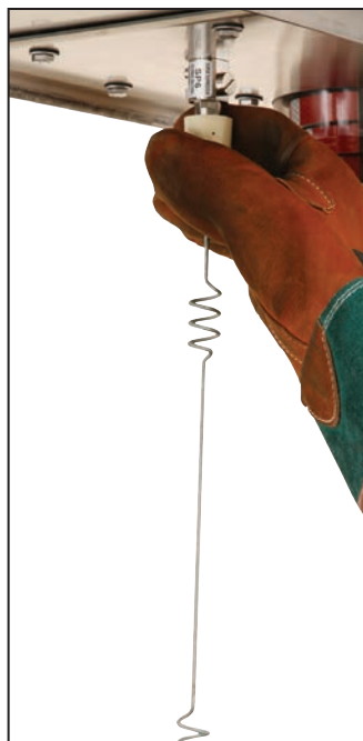
Figure 19. A wire-whip antenna attached to the connector on the bottom of the IntelliRupter fault interrupter base.
