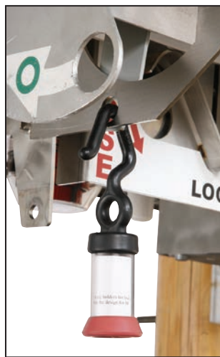
Figure 31. Disconnect open and tagged.
