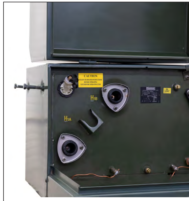
Figure 5. Bushing wells with loadbreak inserts removed.
