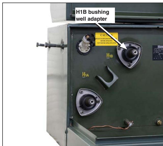
Figure 7. Installed bushing well adapters.
