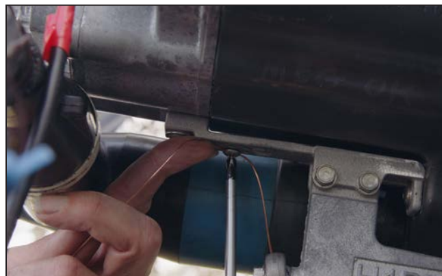
Figure 37. The bushing well interrupter grounding point.
