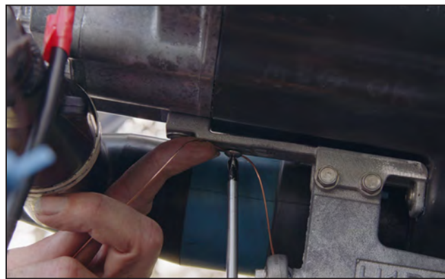
Figure 33. The bushing well interrupter grounding point.
