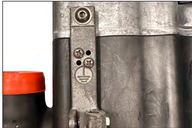
Figure 34. The bushing well interrupter grounding point marked with the "earth ground" symbol.
