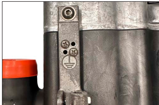
Figure 38. The bushing well interrupter grounding point marked with the "earth ground" symbol.
