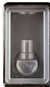
Figure 24. The isolating disconnect after the fault interrupter has been opened and reset.
