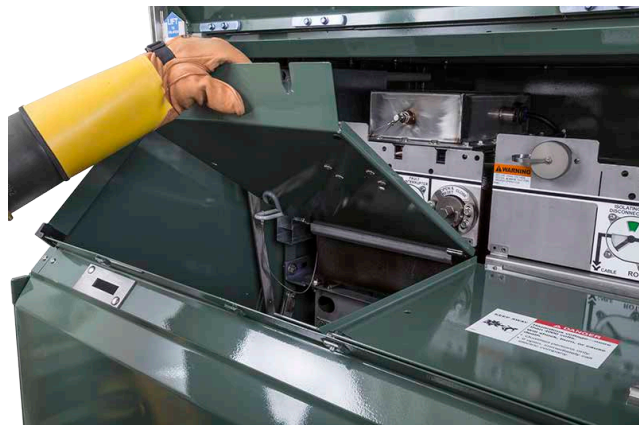
Figure 33. Lift the cover panel to visually inspect the cables or to measure the temperature of the cable terminations.
