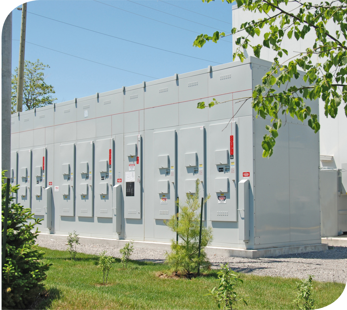
Typical lineup of 46-kV S&C Custom Metal-Enclosed Switchgear.
