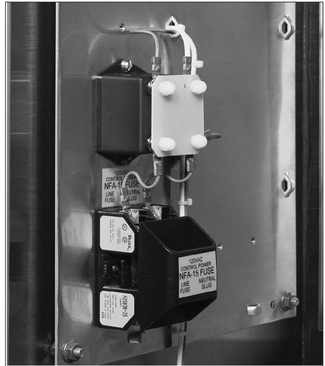
Figure 22. Fuse block for connection of ac control power.
