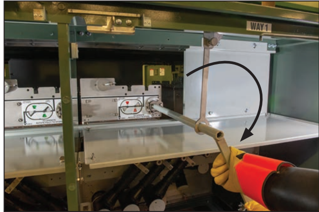
Figure 18. Closing the fault interrupter.
