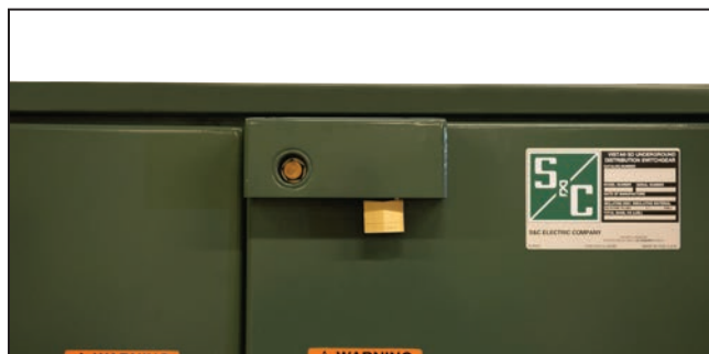
Figure 13. Enclosure doors padlocked.
