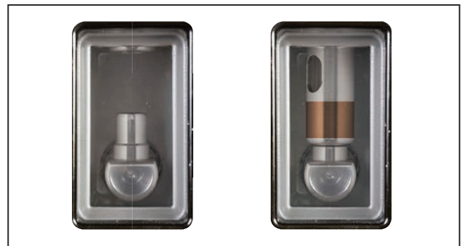
Figure 9. The visible-open gap (isolating disconnect) is easy to see through large viewing windows.
