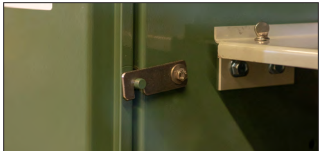
Figure 12. Left door latching mechanism engaged.
