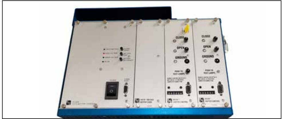
Figure 24. A battery charger with OVER VOLTAGE indicator illuminated.
