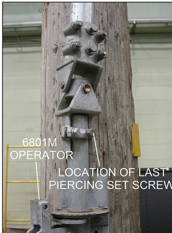
Figure 7. The piercing set screw for the switch operator output shaft is the last to tighten.
