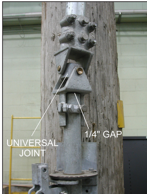
Figure 3. The universal joint showing the 1/4-inch (6-mm) gap for the bottom pipe.
