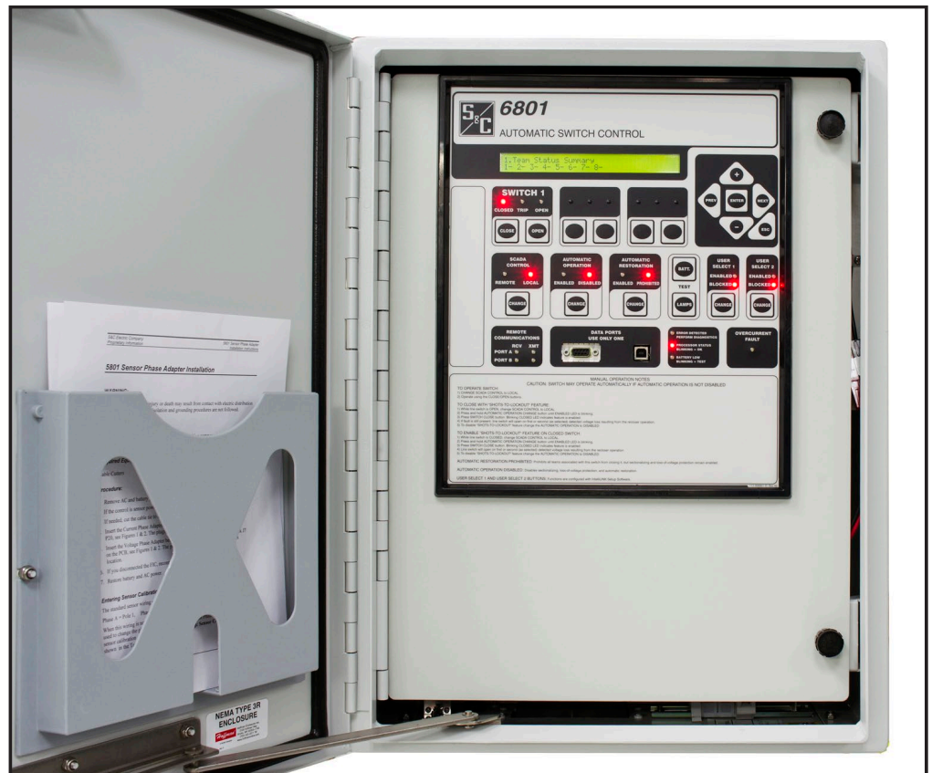
Figure 1. A new 6801 front panel installed on a 5801 control.
