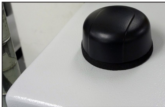
Figure 7. Exterior view of the installed GPS antenna.
