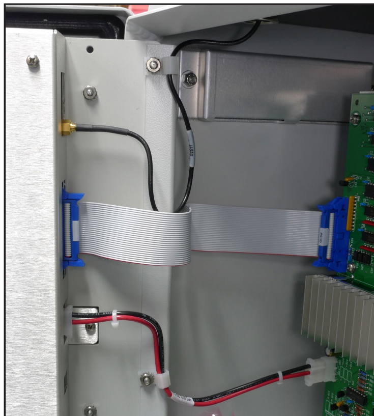
Figure 12. Cables connected to the new 6801 control front panel.
