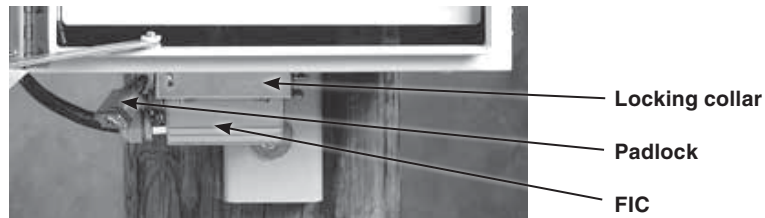
Figure 3. Bottom of switch control enclosure with the FIC connector.
