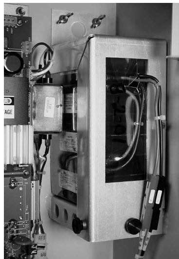
Figure 9. Battery and bracket are on the right, inside the switch control enclosure.
