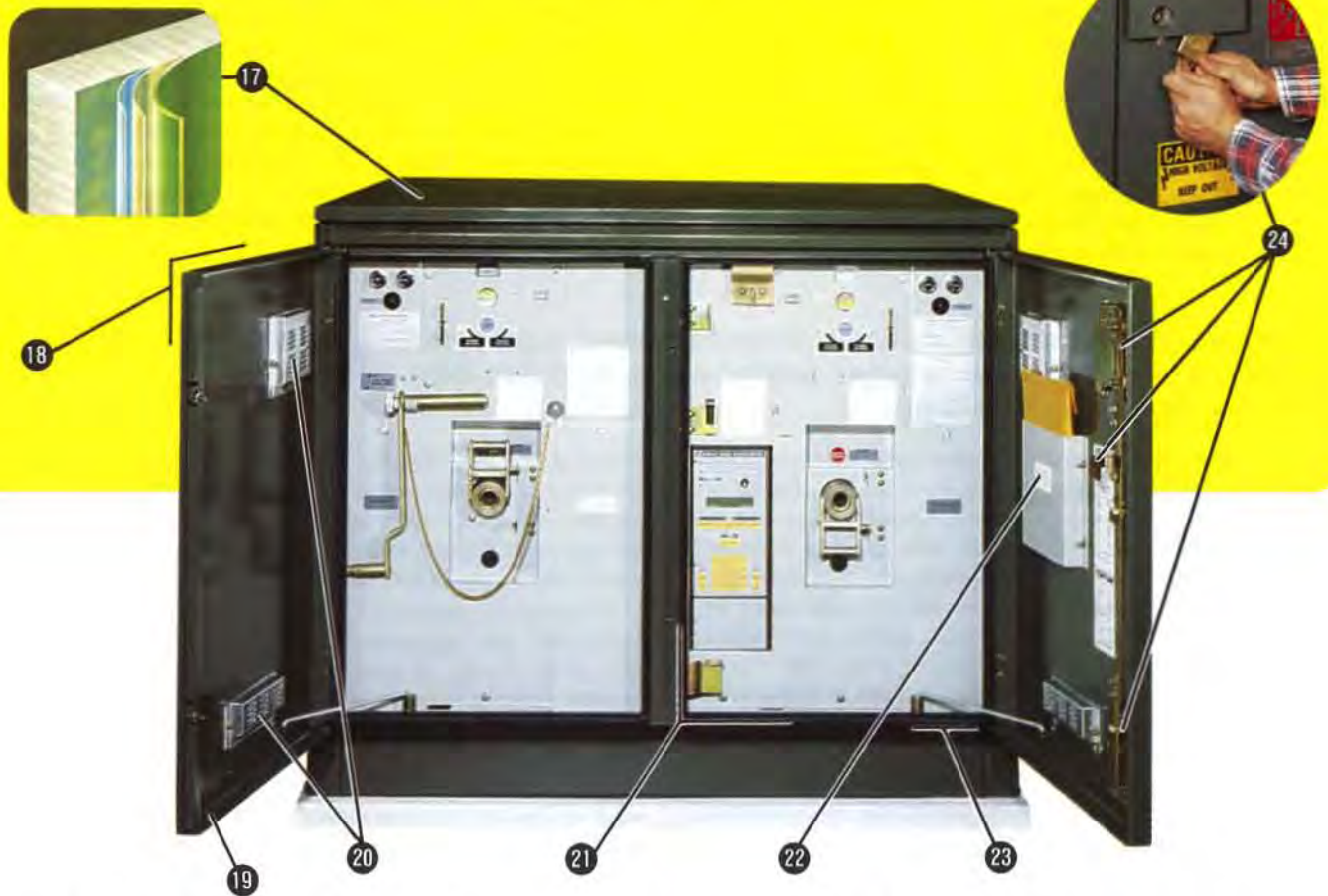
Figure 8. Low-voltage control compartment in source-transfer pad-mounted gear is conveniently located, gives full access to controls without exposure to high voltage.
