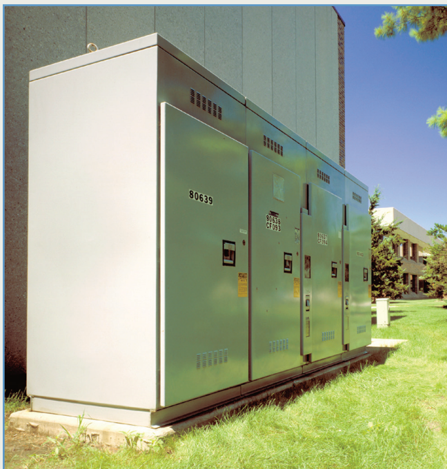
Figure 2. Typical installation of S&C Metal-Enclosed Switchgear with Fault Fiter Electronic Power Fuses.
