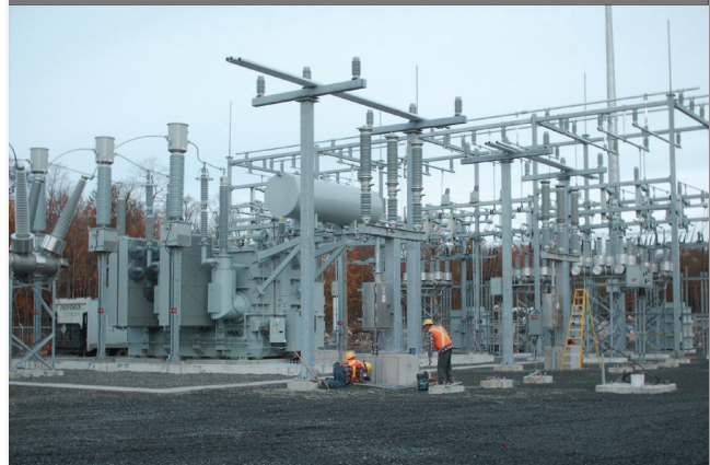
230-kV/34.5-kV Prince 2 Collector Substation.
