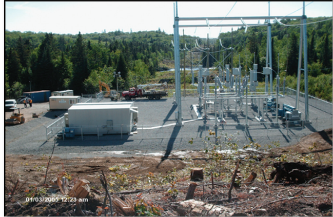
230-kV Heyden Interconnect Substation.
