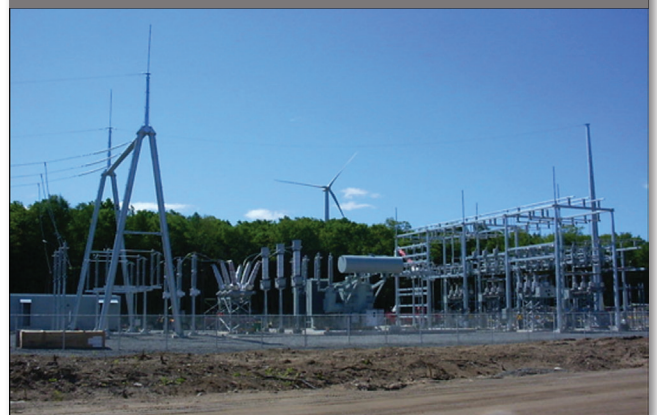
230-kV/34.5-kV Prince 1 Collector Substation.
