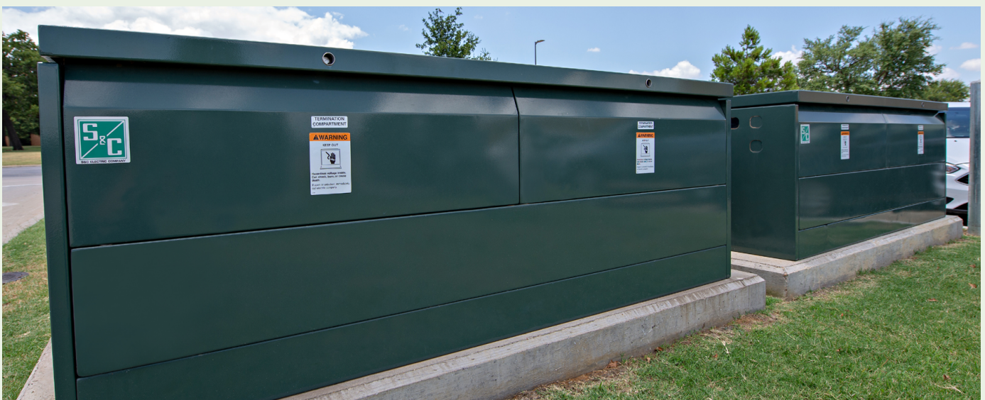
FIGURE 1. Two pad-mount Vista switchgear units.
